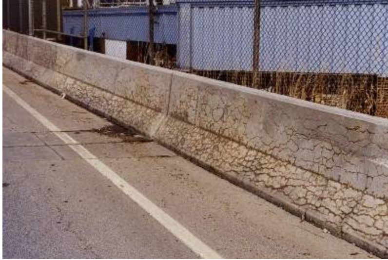
Figure 2.3: Map cracking of ASR affected barrier parapet
