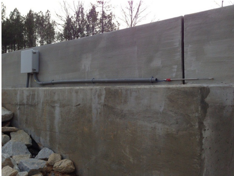
Figure 3.33: VWDG 1 and Enclosure Box 1
