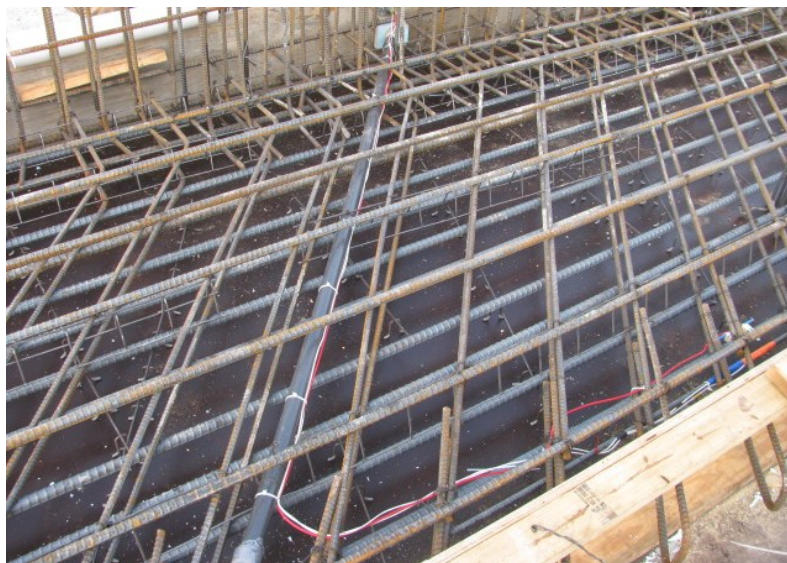
Figure 3.14: Conduit for gage cables
